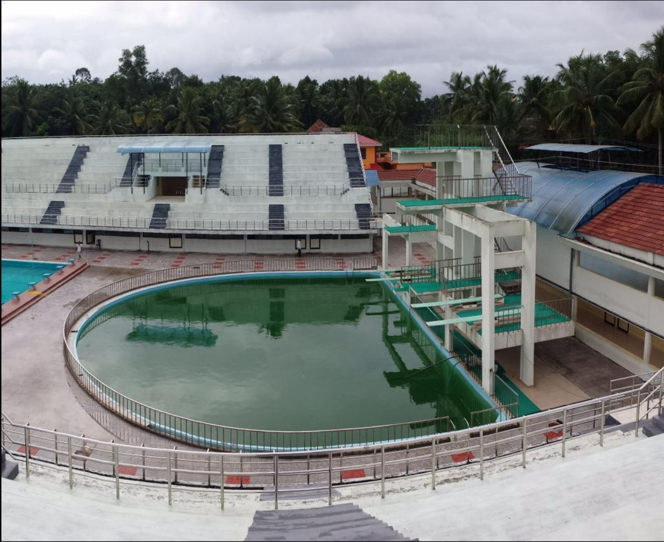
Appendix 1: Photo of Diving Pool at Aquatics Complex, Pirappancode, Thiruvananthapuram
